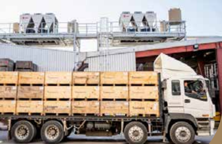
HVAC Units on the roof of Sheds 3 and 4
